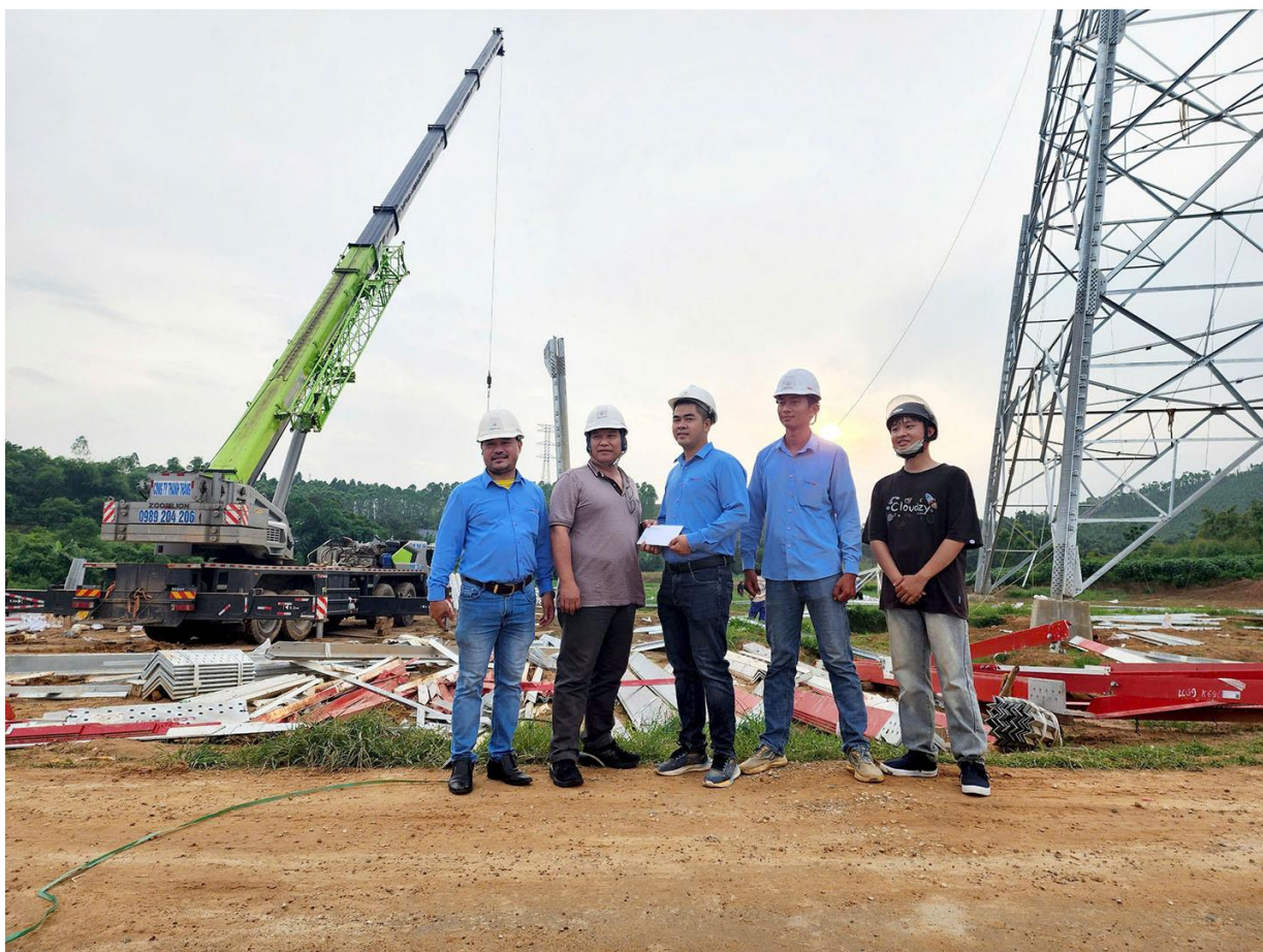
Mr. Le Cao Quyen – Secretary of the Party Committee and Chairman of the Board of Directors of EVNPECC4 – visited and encouraged employees and engaged in supervising the construction of
