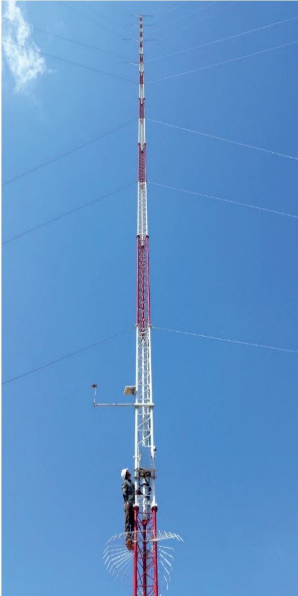
Design, supply, construction and installation of Met Masts; Operating, collecting data and preparing installation report.
